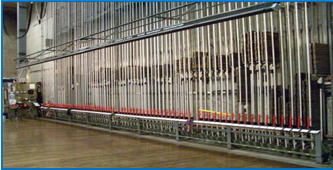
Single Purchase Fly Rail System Stage Right
